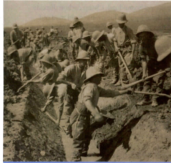
AFTER Troops in Macedonia dig ditches to drain a marsh, part of an effort to eradicate disease-carrying mosquitos.
